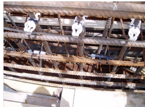
Fig 8: Ribbons of cathodic protection / Rubans de la protection cathodique
