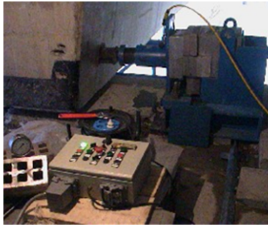
The longitudinal re-centring device. The transversal re-centring device after action, with, in the foreground, the command panel for all operations.
