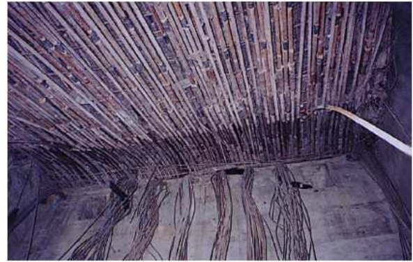
Figure 7. Interior of Airai side a few days after collapse (Photo courtesy SSFM Engineers)
