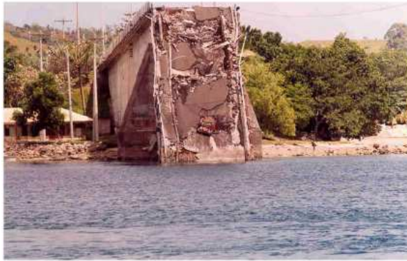
Figure 6. Airai side after collapse.
