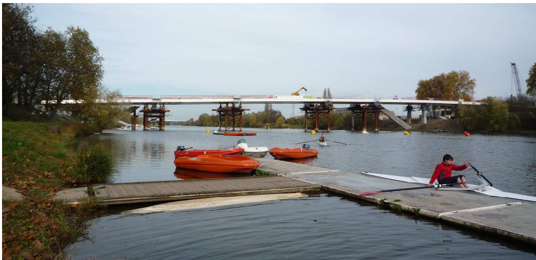
Tablier avant descente sur appuis / Deck before being placed on the substructure
