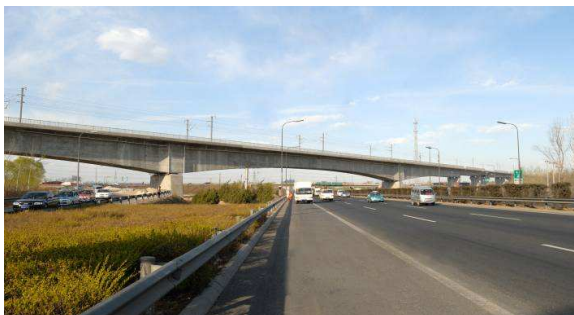
Figure 7 – 5ème rocade – pont à poutre - caisson 80+128+80m 5th ring road - box-girder bridge 80+128+80m
