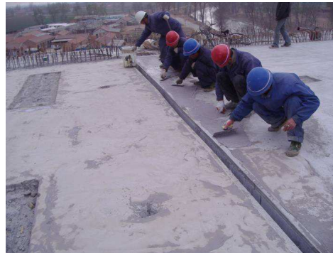
Figure 23 - Repairing the deck surface to achieve the requirements for the relative elevation between adjacent decks
