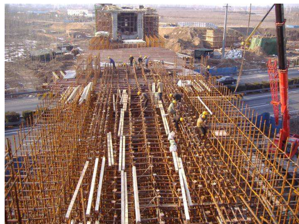
Figure 15 - Installation of scaffoldings over Beijing Ring Road for cast in place continuous bridge Installation d'étais sur la rocade Beijing pour le coulage en place de l'ouvrage continu
