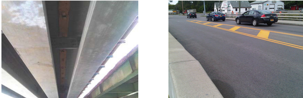
Figure 12 (left) and 13 (right): Canandaigua Outlet Bridge, Village of Lyons, NY, USA (Photos 2012)
