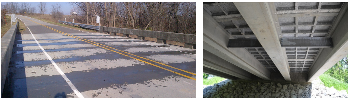
Figure 14: Little Cedar Creek, Wapello County, Iowa UHPC waffle deck bridge with water ponding test (left) and underside view (right)
