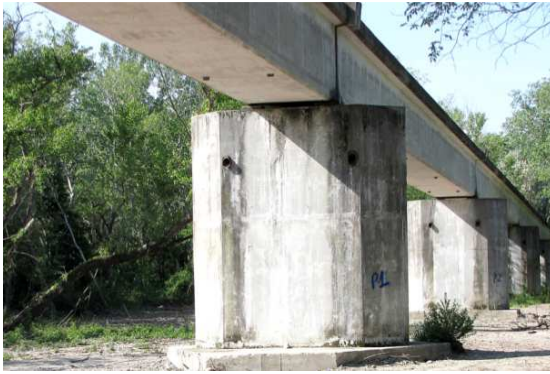
Figure 7 : Vue de la structure avant intervention / View of the structure before the operation
