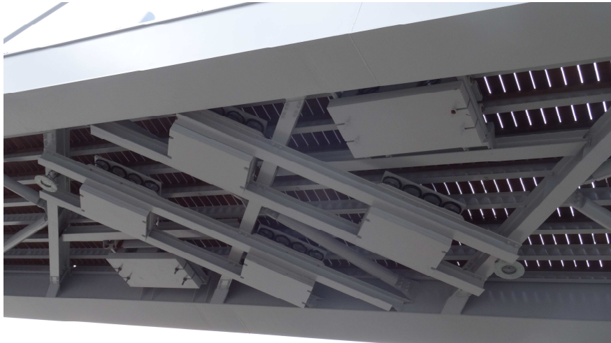
Fig 16: Tuned mass dampers
