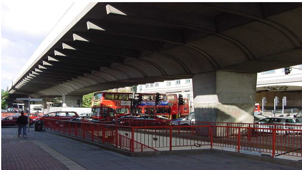
Figure 2: The Hammersmith Flyover before remedial works
