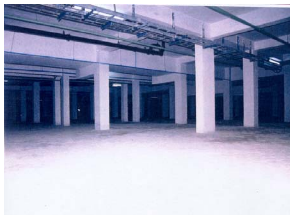
Fig.5: Basement showing service lines
