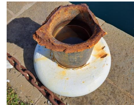
Rupture de bollard
