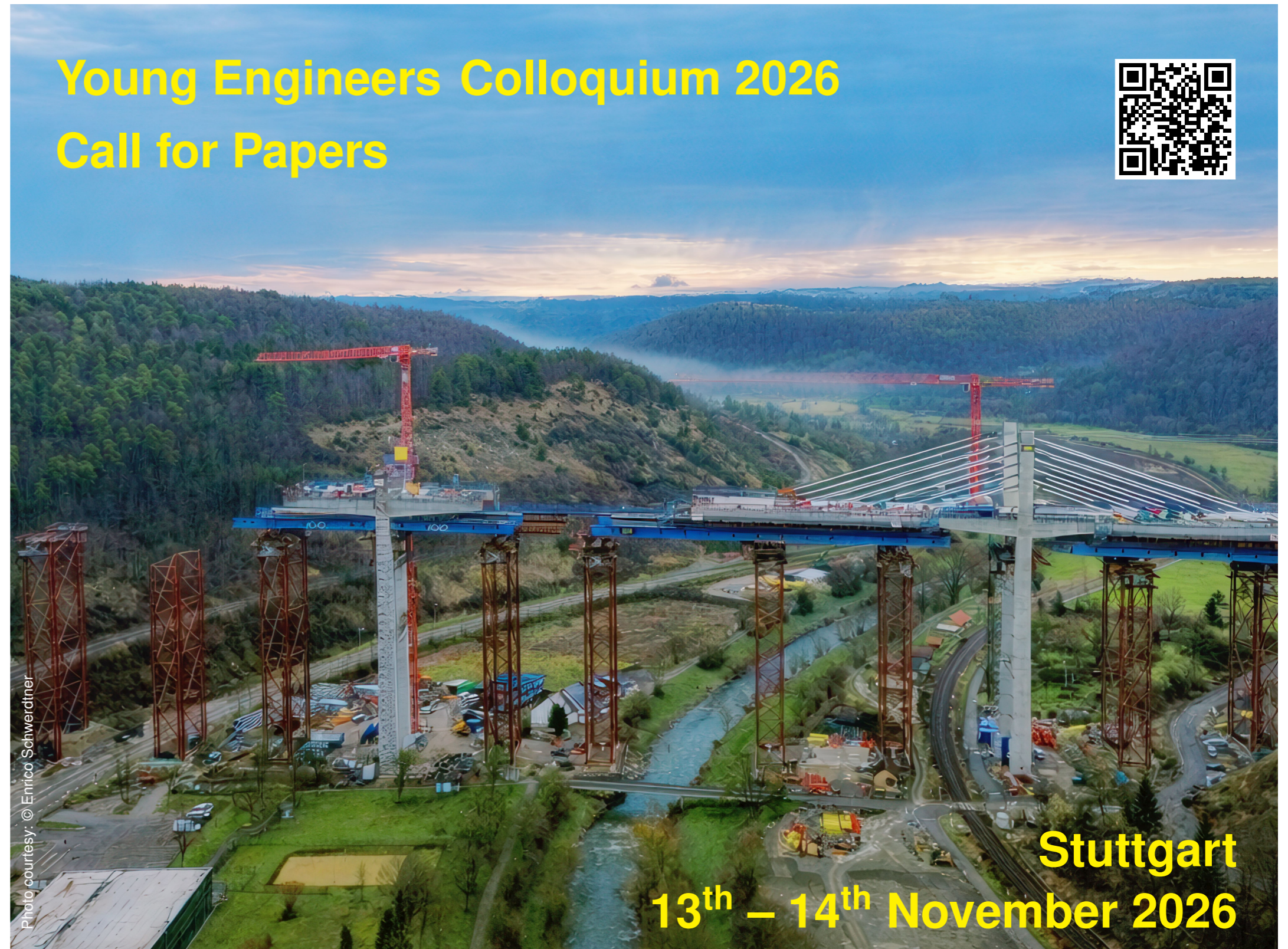
Construction of a new Neckar Valley Bridge along the B32, Horb Bypass, Germany
